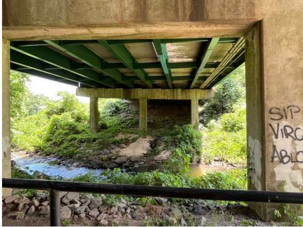
Looking south under I-75 bridge. We would like to have columns across creek painted as well. This can be discussed due to access.
