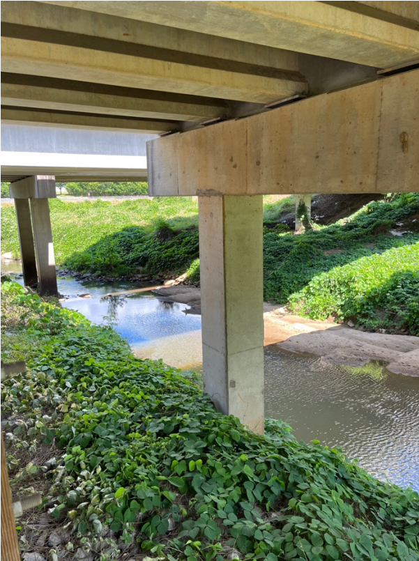
Bridge columns and support. Rock and kudzu on ground level. (Bridge B .) There is a big slope from the trail to the base of the columns.
