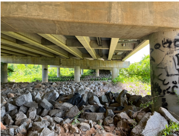
Additional columns and supports. We would like to have columns across creek painted as well. This can be discussed due to access.
