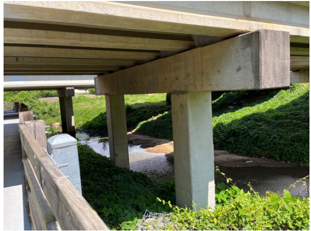
Looking east at I-575 bridge, creek on south side of trail. (Bridge A.)
